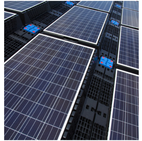
Solar panels on the roof of Bristol City Council's Temple Street office © Bristol Design, Bristol City Council
