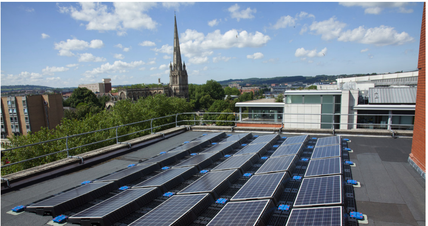
Array of solar panels on the roof of Bristol City Council's Temple Street office © Bristol Design, Bristol City Council
